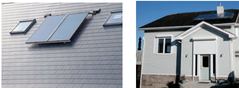
Roof-mounted Solar Collectors for domestic hot water system 4
